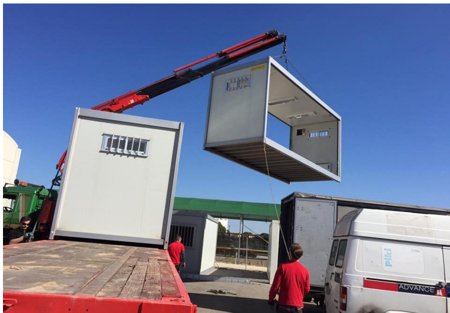
Figure 9.1 — Transport, lifting and on-site installation of CLT modules, enabling rapid assembly with minimal disruption.
